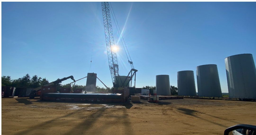
Wind turbine assembly at Tobique First Nation as part of the Wocawson Project Photo courtesy of Tanna Pirie
